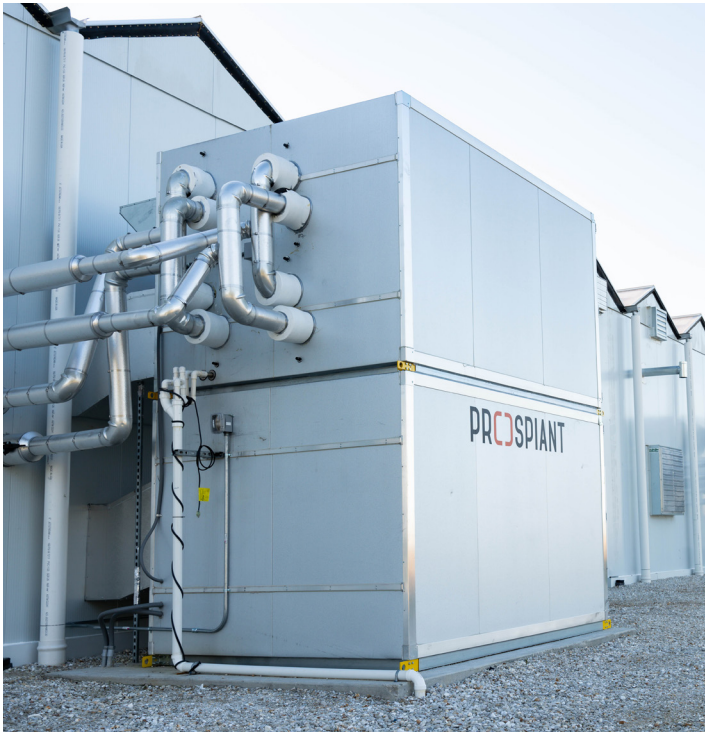
Exterior Air Handling Unit
