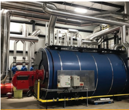
Large hydronic heating system with CO 2 recovery
