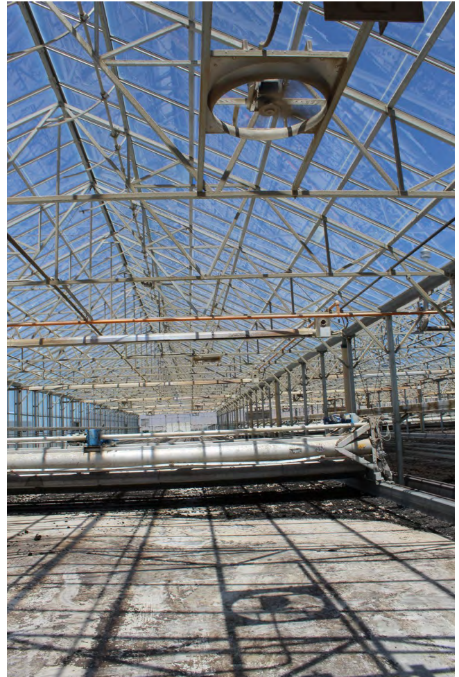
Controlled vertical airflow using reversible VAF fans helps prevent humid air from lingering near the sludge surface.
