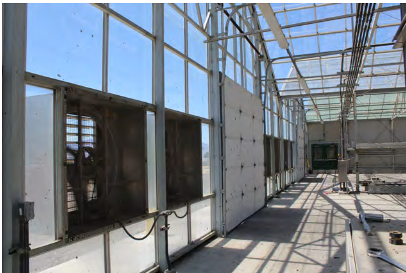
Exhaust fans pull moisture-laden air out of the greenhouse to make room for drier outside air.
